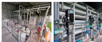
Filtration equipment used in wastewater treatment.
